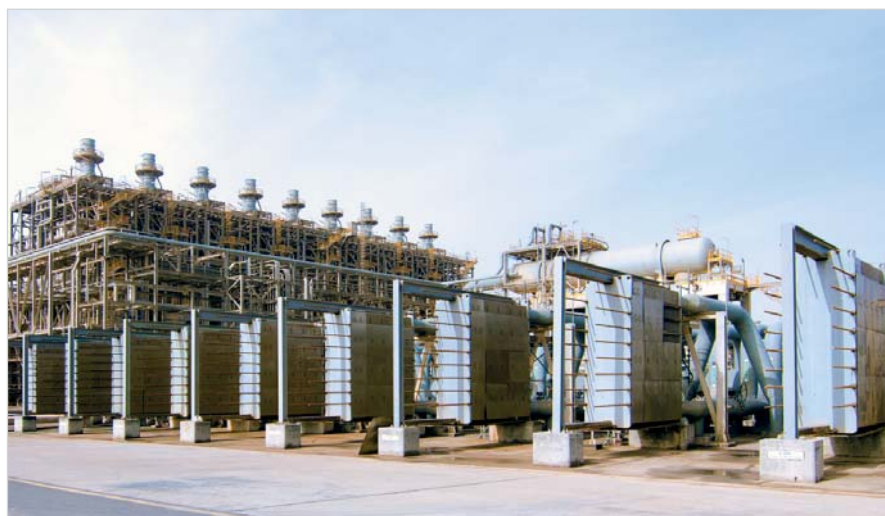
SPX APV plate heat exchangers at Ras Laffan, Qatar. Photo courtesy Ras Laffan Olefins Company (RLOC)
